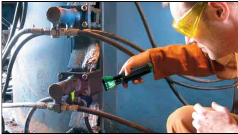
Leak checking valves and fittings with the OPTIMAX™ 3000 blue light LED flashlight
